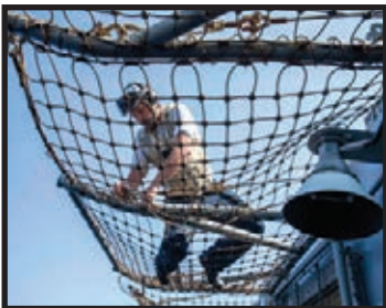
Debris Fall Nets
